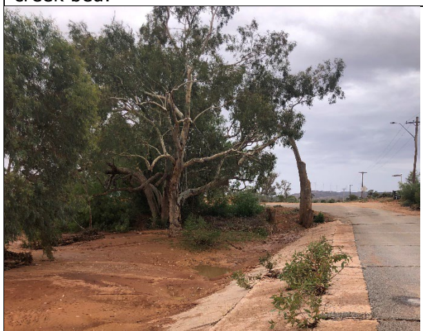
Photo 5: Penrose Park Road causeway with sand build up on the downstream site
